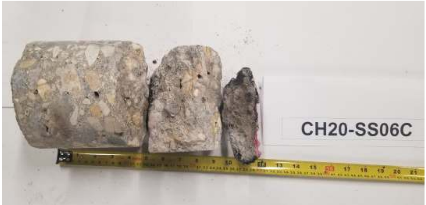
Granular Structure Below Pavement: Gravel fill – sandy, poorly graded, fine grained, damp to moist, compact (inferred), light brown
